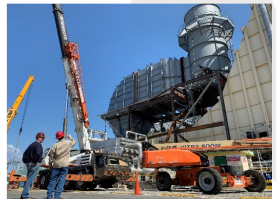
Bypass Stack (one day before startup)
